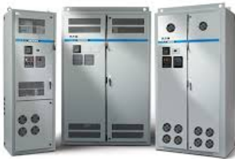
VARIABLE FREQUENCY DRIVERS (VFD)/ SOFT STARTER CONTROL TECHNIQUE (NIDEC)
