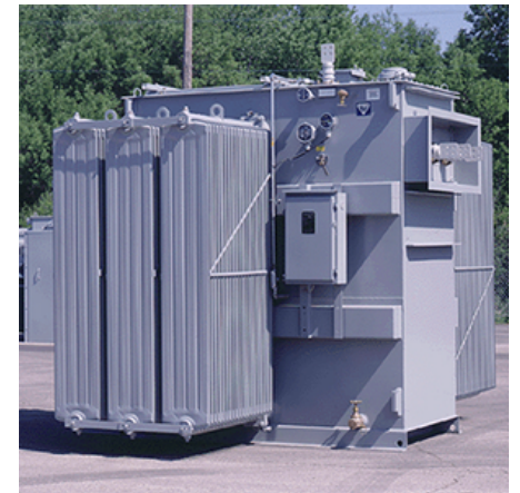
ELECTRICAL TRANSFORMER (SUBSTATION)
